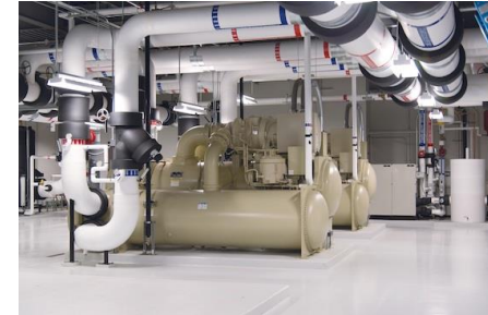
(Photo: Chiller & Cooling Best Practices)
